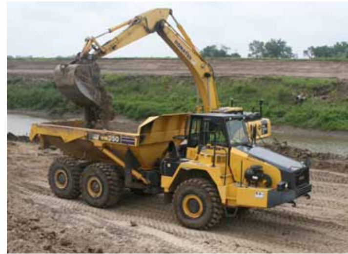
Ebert Construction uses an excavator to load one of two articulated haulers on the north side of Soldier Creek.
