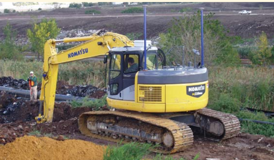
▲ A machine operator from Edgeboro International installs gas collection piping using an excavator-mounted AMG system at the Kingsland Landfill.
