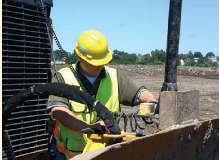
▲ At the Avon Landfill in Lyndhurst, Stephen Stafniak, PLS replaces a dual-axis tilt sensor mounted on the blade of a bulldozer.
